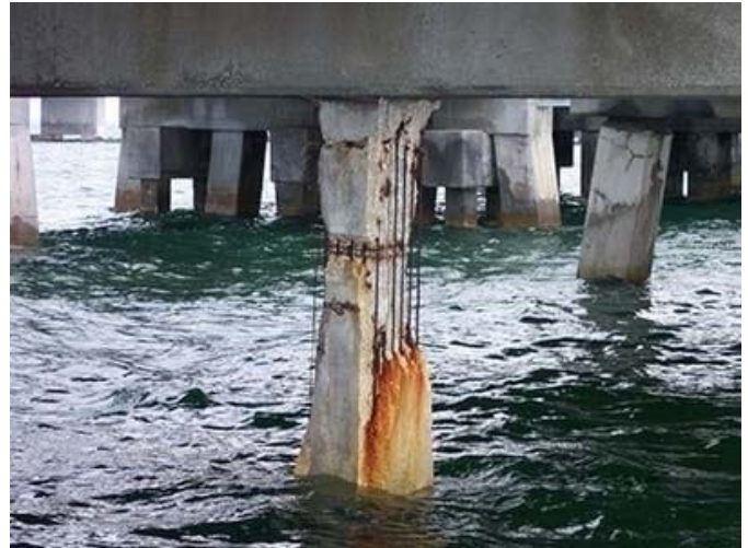
Steel corrosion to rebar in concrete pier
