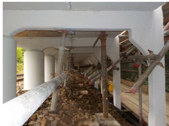
External columns fitted with new reinforcement and micro porous concrete to strengthen the Railside columns of this platform.
