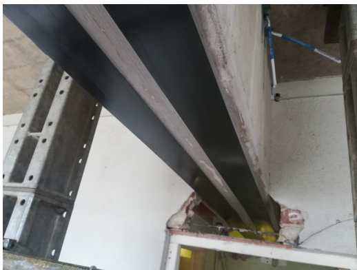
Carbon fibre solid strips used to underside of concrete beam to strengthen flexural movement
