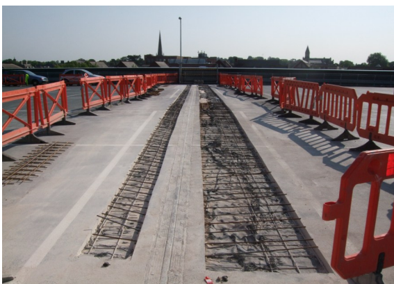
Additional reinforcement added to existing floor slab to extend existing mesh to reach the full slab width.
