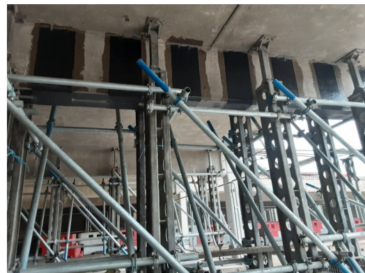
Carbon fibre mesh wrapped around beam to secure beam to floor above.
